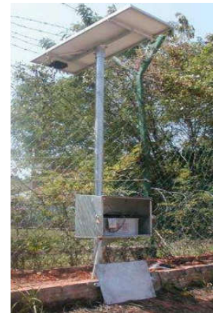
With Solar Power on site picture.
